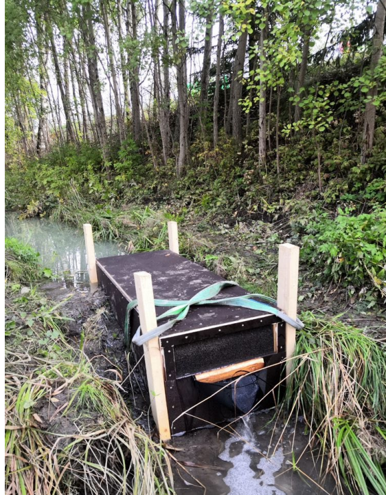
Fig15. Testing of the first filter prototype. View from downstream/outlet side.
