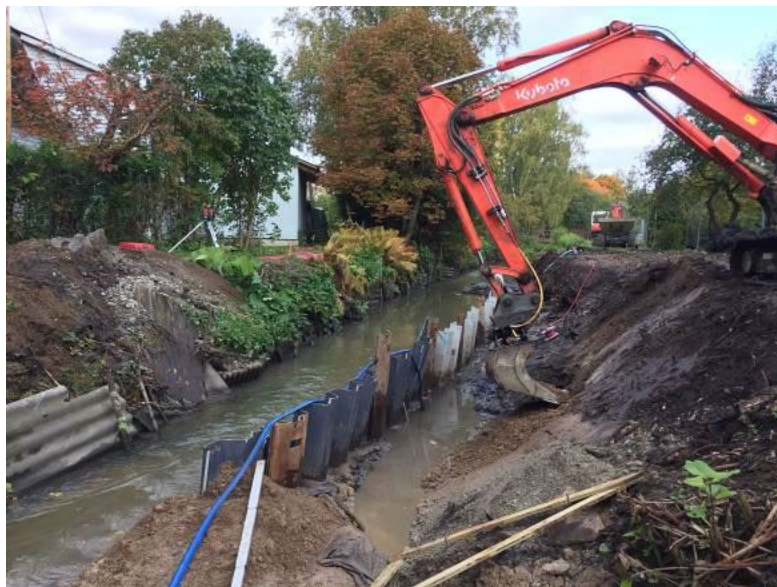
Fig. 5: Use of cofferdams to keep parts of the river bed and banks dry for construction works.
