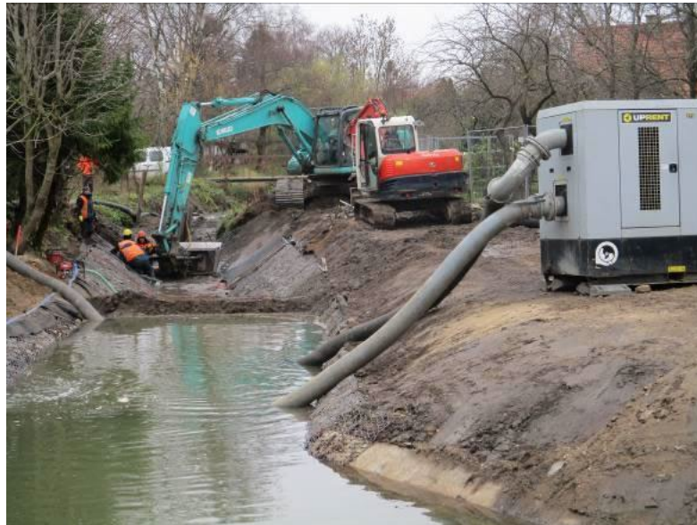
Fig. 6. Section of the river were dammed and drained with two large pumps.
