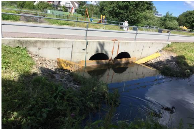
Fig. 8: Blocking of a road culvert to keep the downstream section of the river dry for the period of a few hours to allow for construction works.
