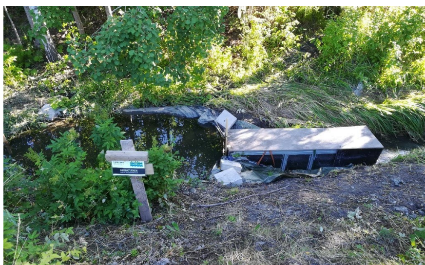
Fig. 26. Final stream filter deployed and in operation. The filter was covered with plywood to protect it from vandalism at the pilot site.
